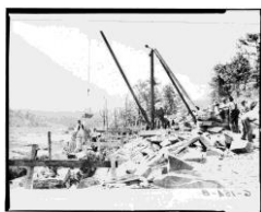
Title: 226. Early construction on section 2-A-1. This was the site of the first construction on the Blue Ridge Parkway. - Blue Ridge Parkway, Between Shenandoah National Park & Great Smoky Mountains, Asheville, Buncombe County, NC
